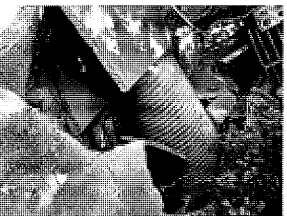
COLLAPSED BRIDGE/PIPE BLOCKING CREEK
